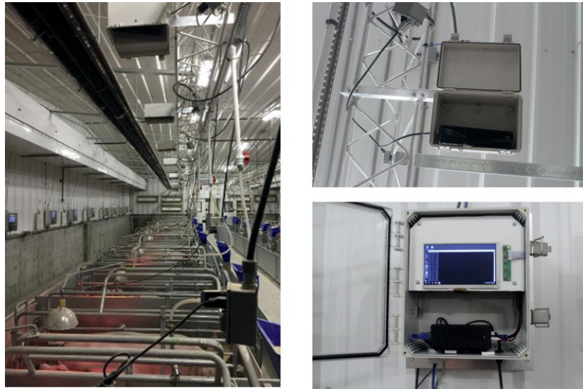
Figure 1: Shows the installed system with Kinect V2™ mounted on aluminum truss
